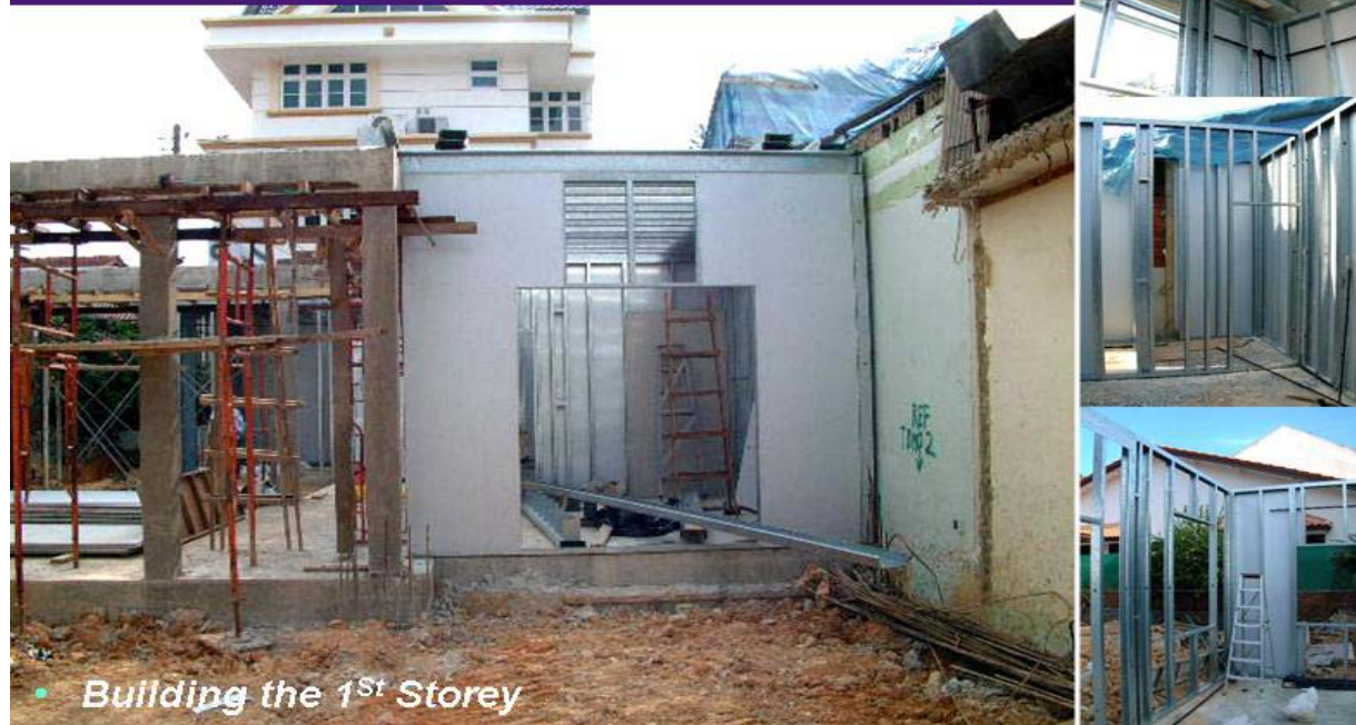
Figure 12.11 Construction of first storey. Only the front panel used CIS construction, all other areas used light gauge steel frames
