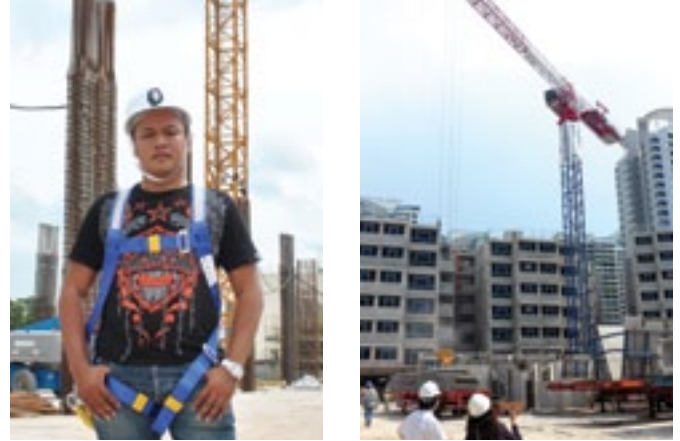
Top Left | Mr Imran, a licensed tower crane operator, at his new commercial project in Woodlands.
