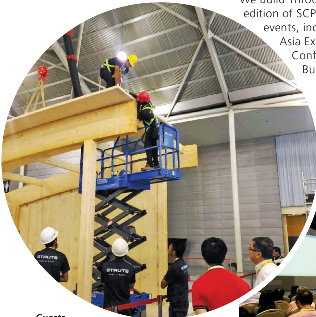
Guests observing a demonstration at the Skilled Builders Project, which featured the installation of a curved roof, MEP systems, air con fabric duct, and architectural finishing works like drywall and laminated flooring.
