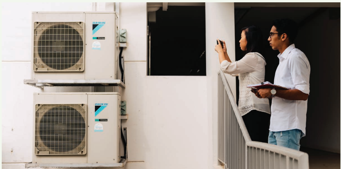
Checking the energy performance of air conditioner units.
