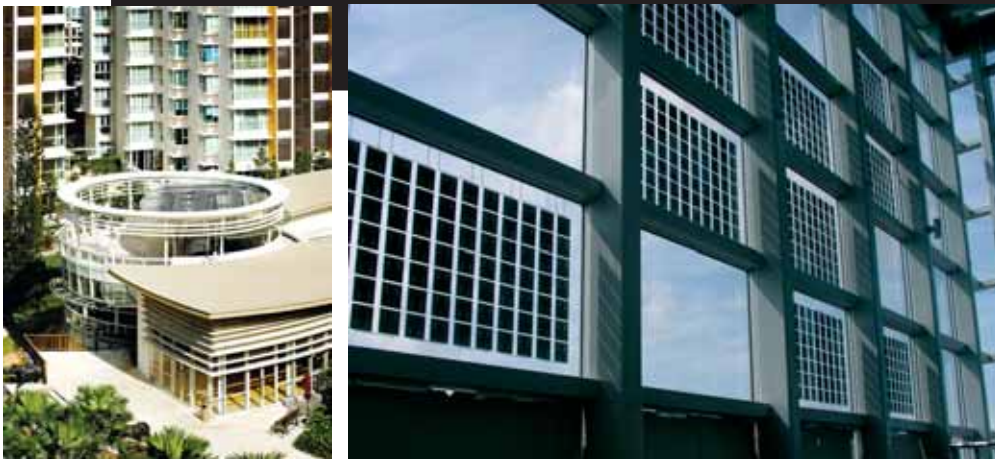
Photo Voltaic installations in Savannah CondoPark and Biopolis
