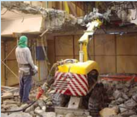
Purchase of equipment such as remote-controlled demolition equipment to facilitate improved resource recovery. (Photo credit: Brokk)
