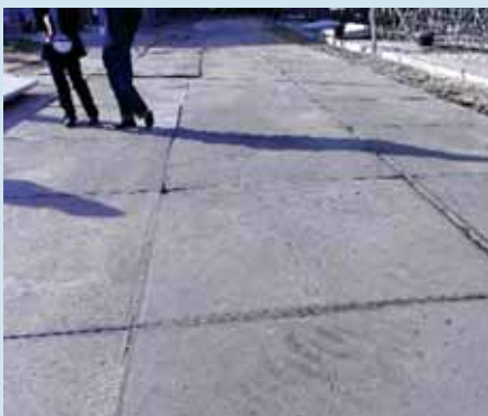
Test-bedding to study feasibility of alternative materials such as using soil hardeners or precast slabs to construct temporary roads.
