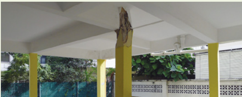
Top | Serious spalling of concrete.
