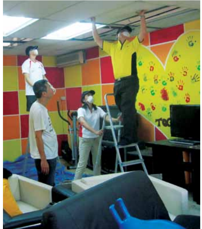
Right | With BCA's Group Directors Mr Koh Lin Ji and Ms Jeanna Das helping to replace the ceiling boards at SAVH's Recreation Room.
