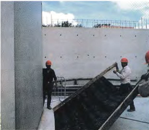
Off-form finish requires attention to mould precision, casting, demoulding and surface protective coating
