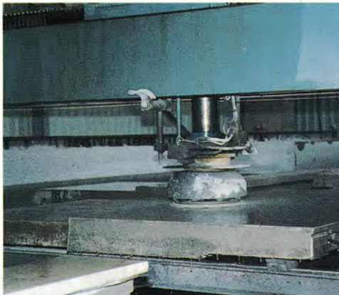
Polishing of concrete panel to give a highly polished surface similar to stonework
