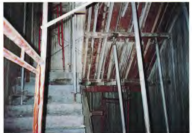
Scaffolding and formwork constitute a high percentage of preliminaries for cast in-situ projects
