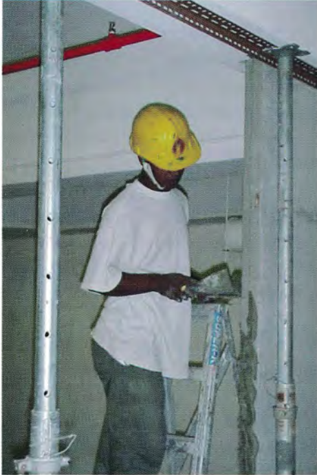
Installation of precast hollow core panel: Using temporary angle as a guide for alignment of wall
