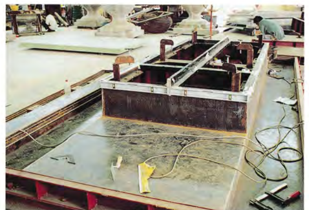
A recessed window precast facade using steel mould, aluminium window frame is cast together to provide a weather-tight joint
