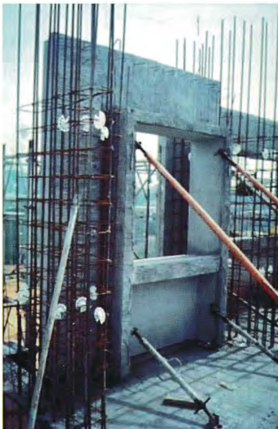
HDB precast facade being prepared for 'Wet' joint connection with in-situ column
