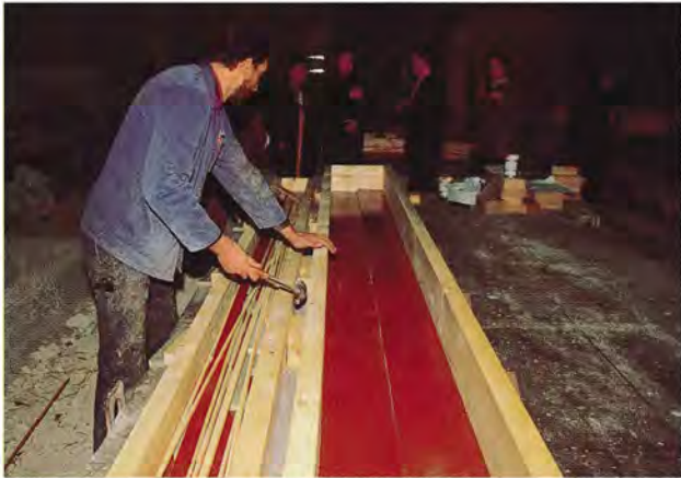
A mould for a large precast parapet wall panel under construction. In France, moulds are frequently constructed from high grade softwood which allows substantial alterations to be made relatively easily
