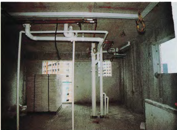
Pipings ready for the pre-assembled toilet unit
