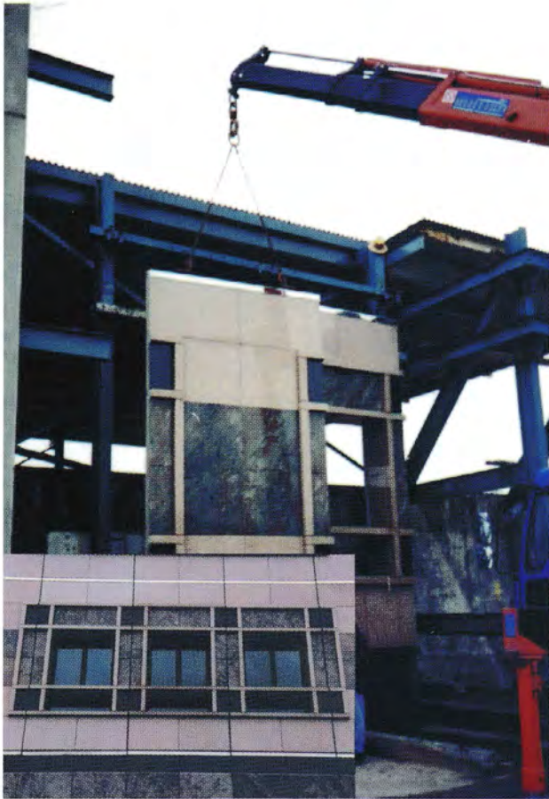
Inland Revenue House Singapore: The ribs are solid granite inserts to create a patterned feature. Different coloured granites have been used to add visual interest to the external precast wall
