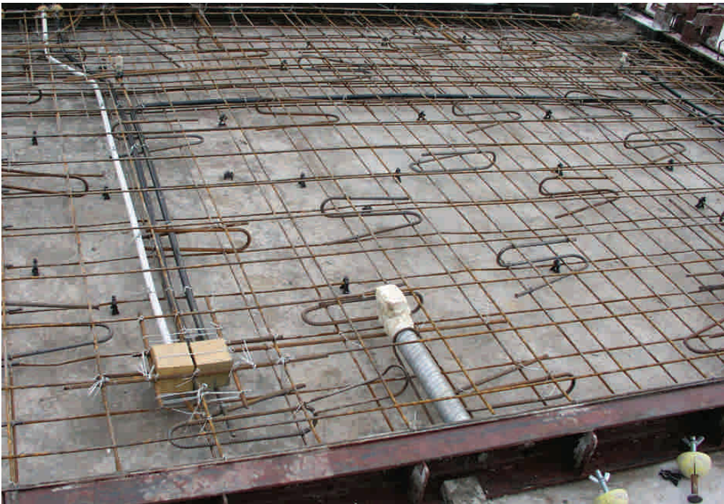
Fig. 3.2 – Cast in conduits for electrical services within the wall panels
