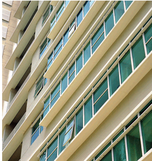
Fig. 6.45 – Deep profiled precast bay windows, sun-shading ledges for aesthetic and functional purpose
