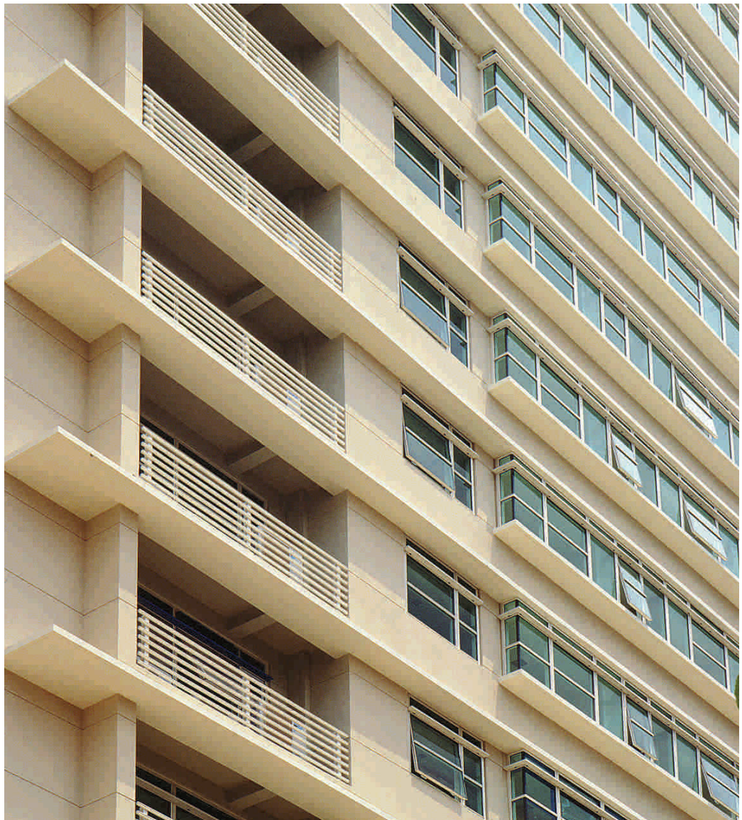
Fig. 1.15 – Horizontal and vertical grooves line together with joint details can be part of the architectural feature
