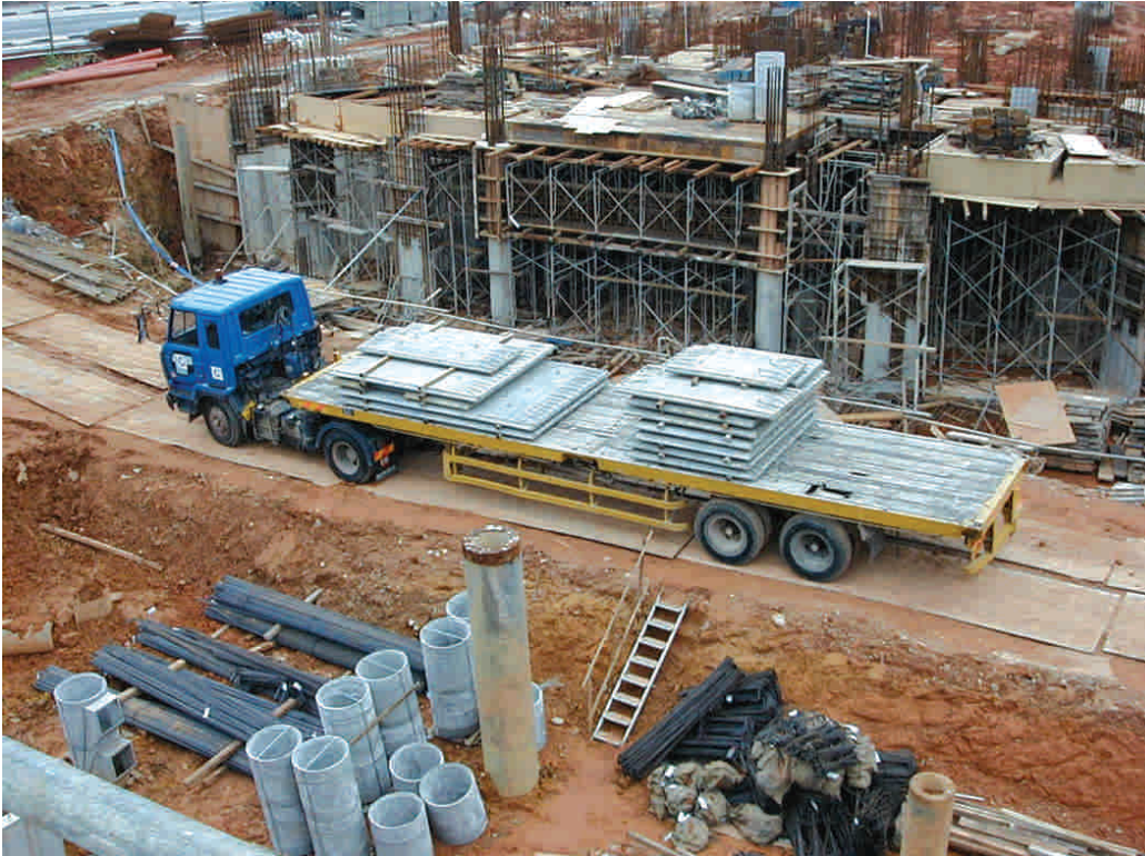
Fig. 4.1 – Site access is important for the delivery and erection of precast components
