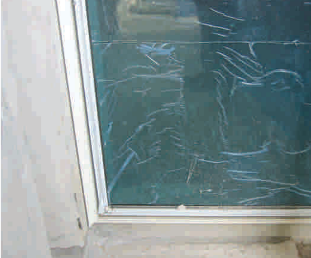
Fig. 1.20 – Tolerances/ gaps between the precast column/ beam and the window unit are required
