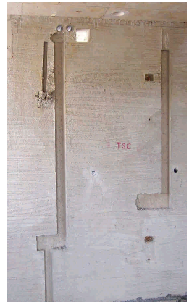
Fig. 6.15 – Recesses incorporated in precast wall to conceal M & E services at later stage
