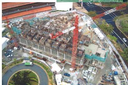
Fig. 6.19 – The Jade under construction Two tower cranes were deployed for the site construction
