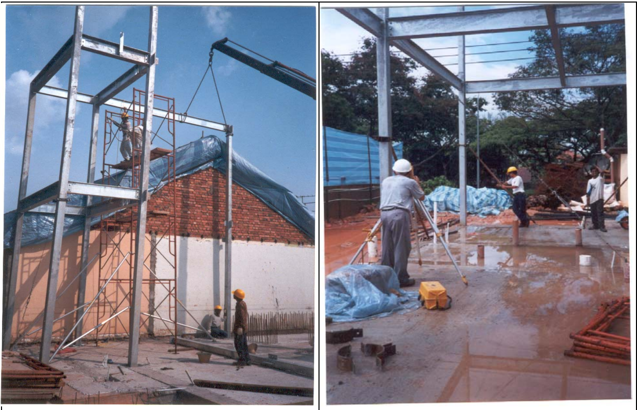
Figure 8.1 Erection of steel column and beams - Temporary bracing was required to ensure verticality of steel columns when bolt connections from beams to columns were tightened.
