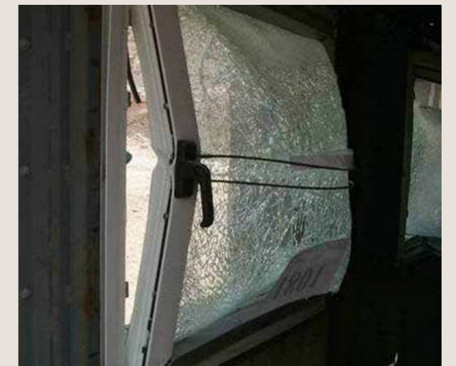
Figure 42: Window after explosion
