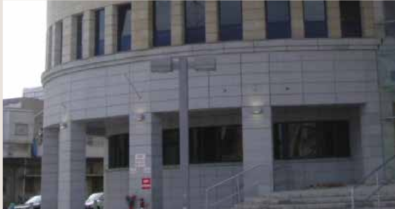
Figure 18: Example of external wall with exposed column line - poor design
