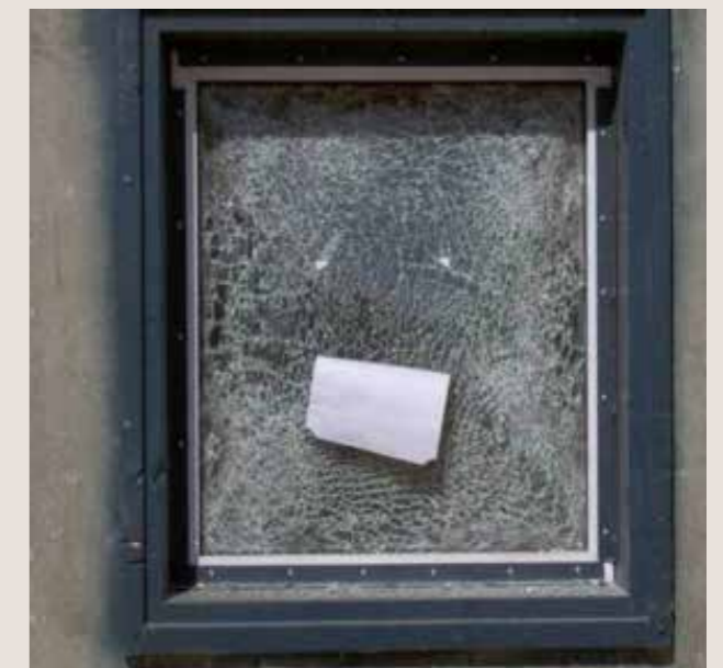
Figure 31: A window protected by mechanically anchored ASF for basic blast level (after explosion)
