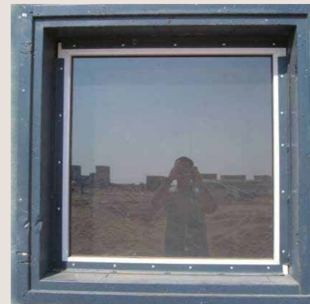
Figure 30: A window protected by mechanically anchored ASF for basic blast level (before explosion)
