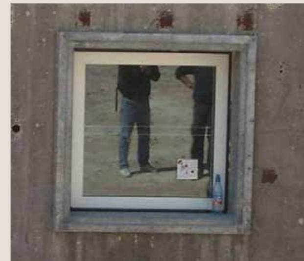
Figure 41: Window before explosion
