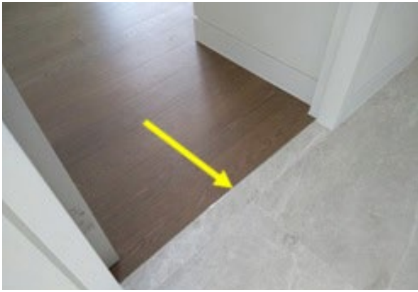
Joint with metallic strip
