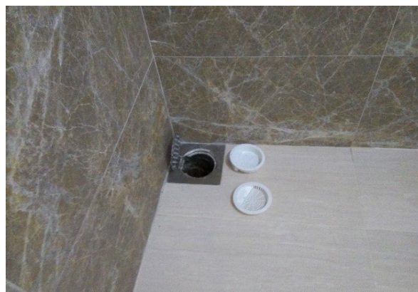
Joint at floor trap covered with grout
