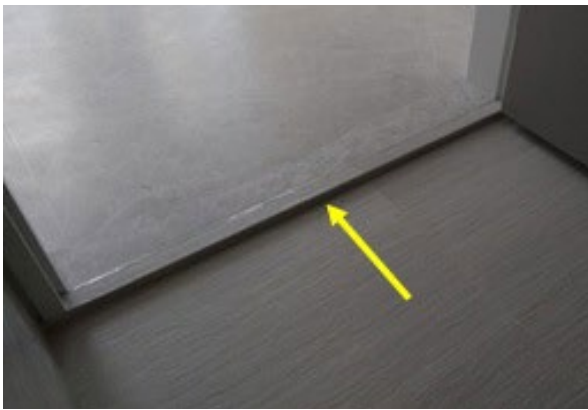
Threshold to reduce water ingress
