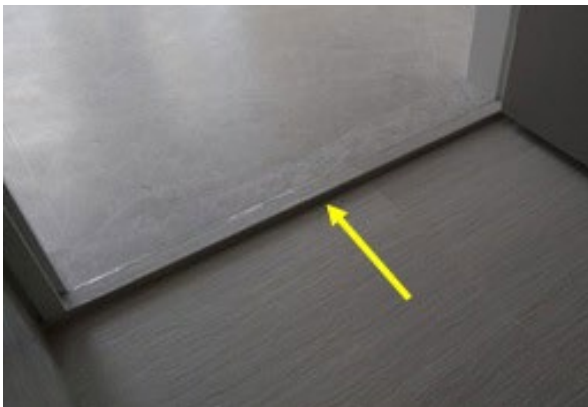
Threshold to reduce water ingress
