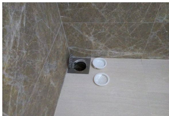
Joint at floor trap covered with grout
