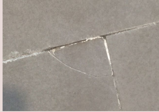
Cracks Figure 5.5.n
