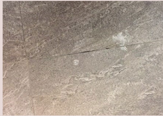
Paint stains Figure 5.5.f
