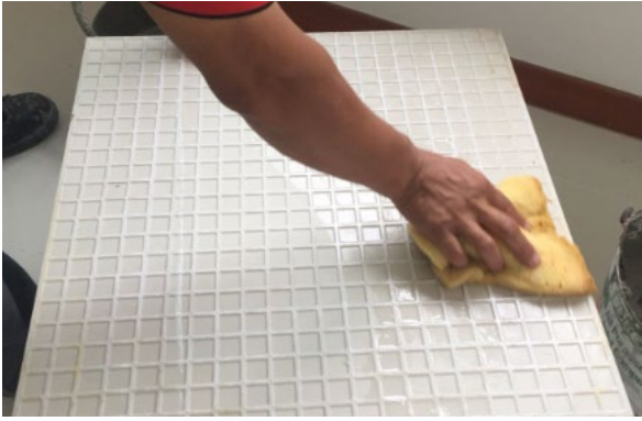
Cleaning ceramic tile to remove dirt and dust before laying Figure 5.2.a
