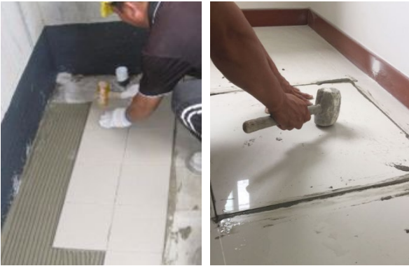
Using mallet to tap on tile for good coverage of tile adhesive between tile's back and floor substrate Figure 5.2.e
