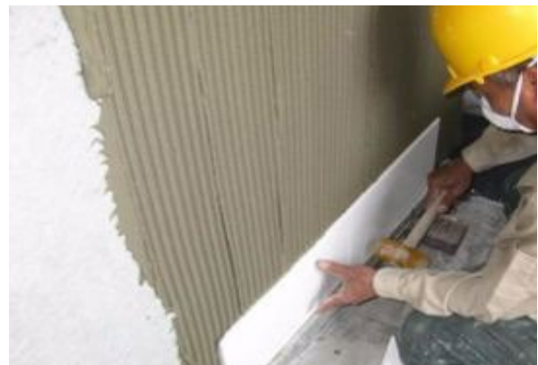
Using rubber mallet to tap on tile after laying for uniformity Figure 5.2.l
