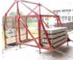
Travellator Hanging Platform
