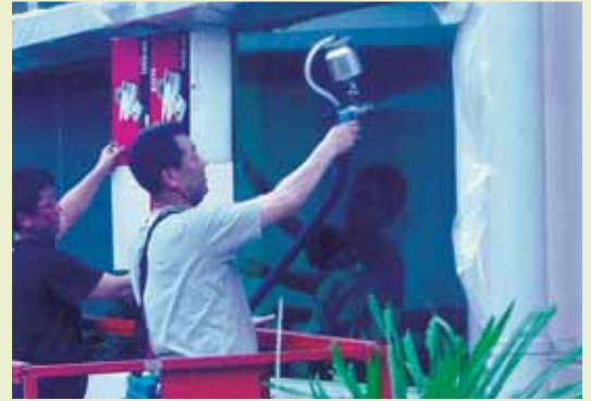
Workers spraying on the heat insulation coating for glass at BCA Academy.
