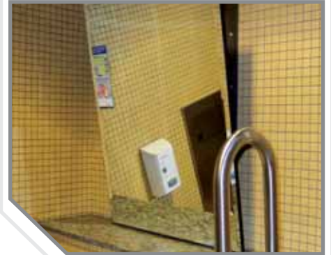
Tilted mirror in accessible toilet
